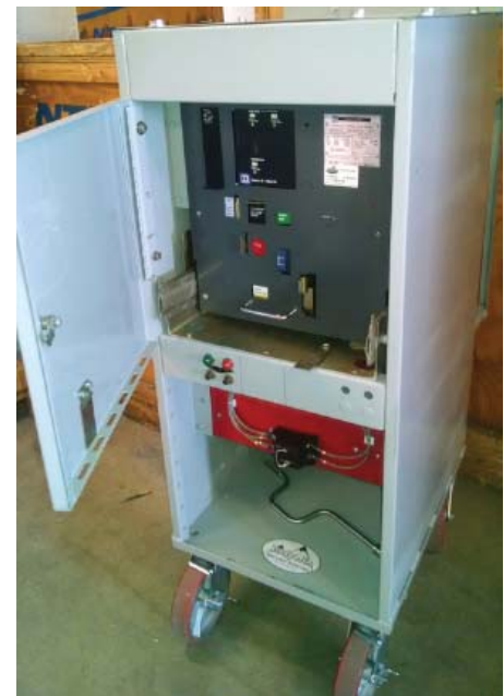
CAPTION: The Eaton DS Low Voltage Power Circuit Breaker (formerly Westinghouse) is a modern air circuit breaker commonly used in distribution systems throughout industry. The 800 Amp frame size breaker supplied for class is operated both electrically and mechanically and is fully rackable in a mock cubicle with an infrared window, bus work and control power.
